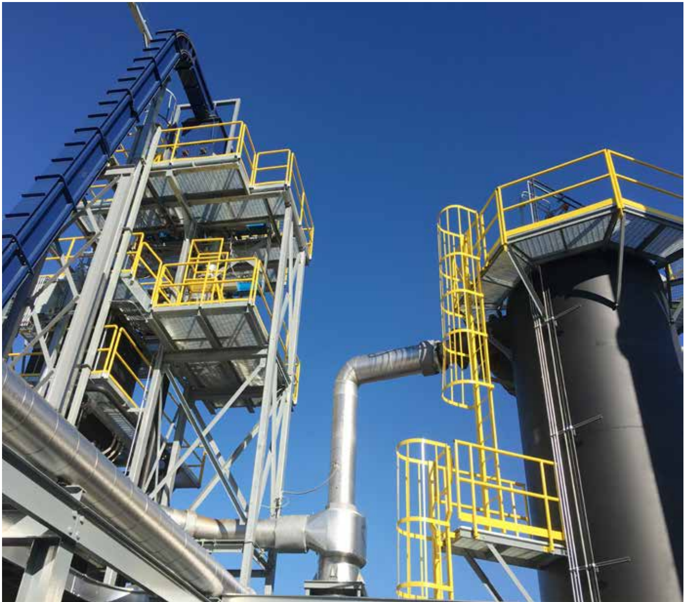
In addition to the downdraft gasifier, on the left, the City of Lebanon's gasification facility includes a thermal oxidizer, on the right. Aries Clean Energy
